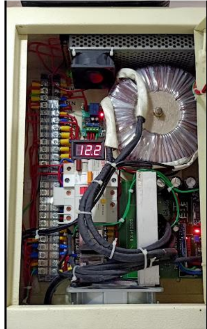
Gambar 7. UPS ( Uninterruptible Power Supply ).
